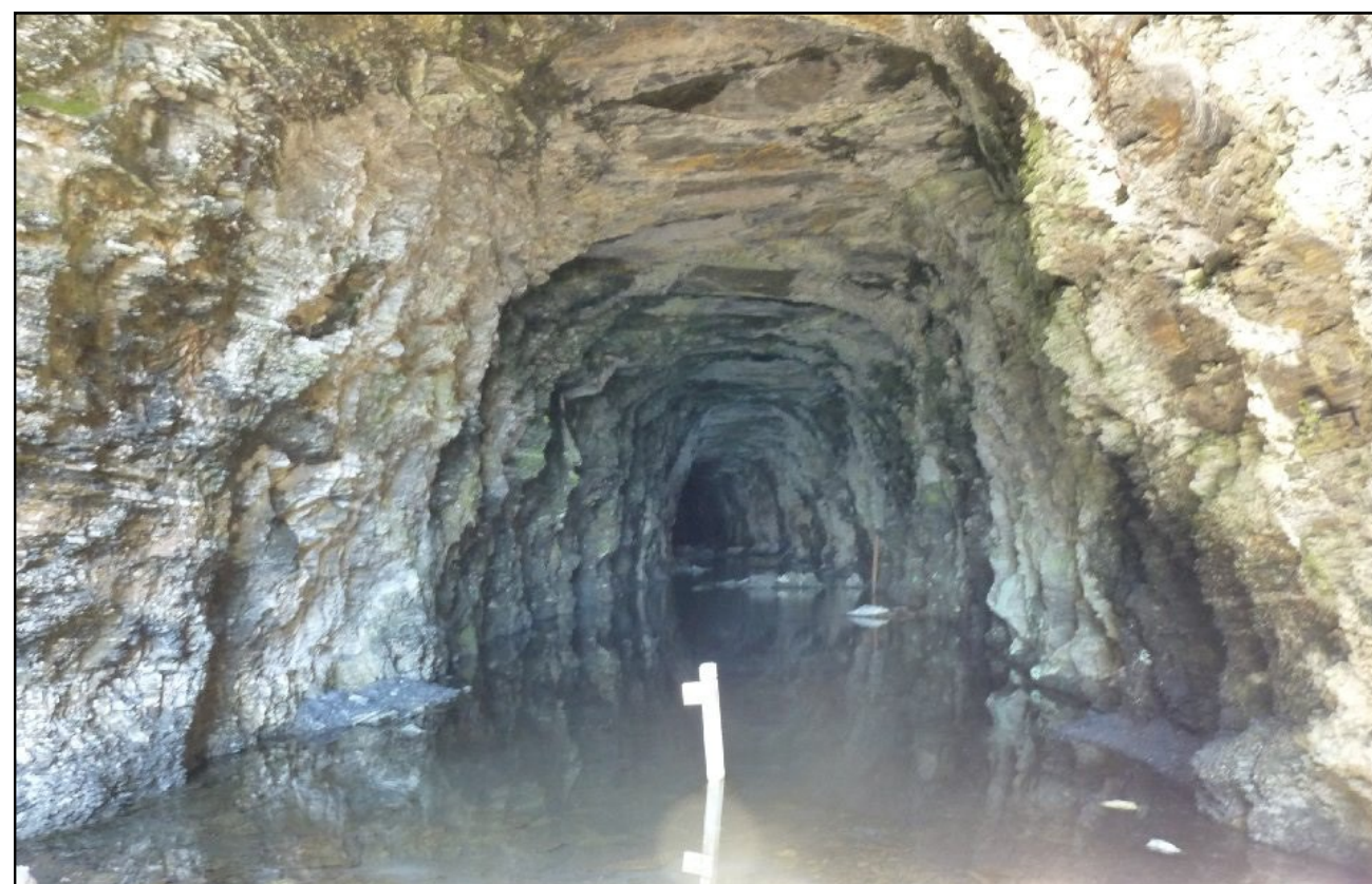
Close-up of the southeast portal of the High View tunnel showing gently west-dipping bedding, water in tunnel (a constant problem during railroad operations), and lack of lining at portal.
