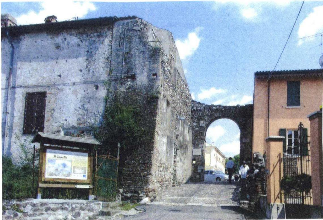
More presently-visible battle damage at Solferino: shell holes in building wall outside entrance to Piazza Castello / castle square (very difficult to notice, because the steep road up from the village comes to a 4-way stop with no visibility to the right or left-behind, and you have to drive across and turn normal-left to go through this narrow gate/arch without scraping its sides). Br91
