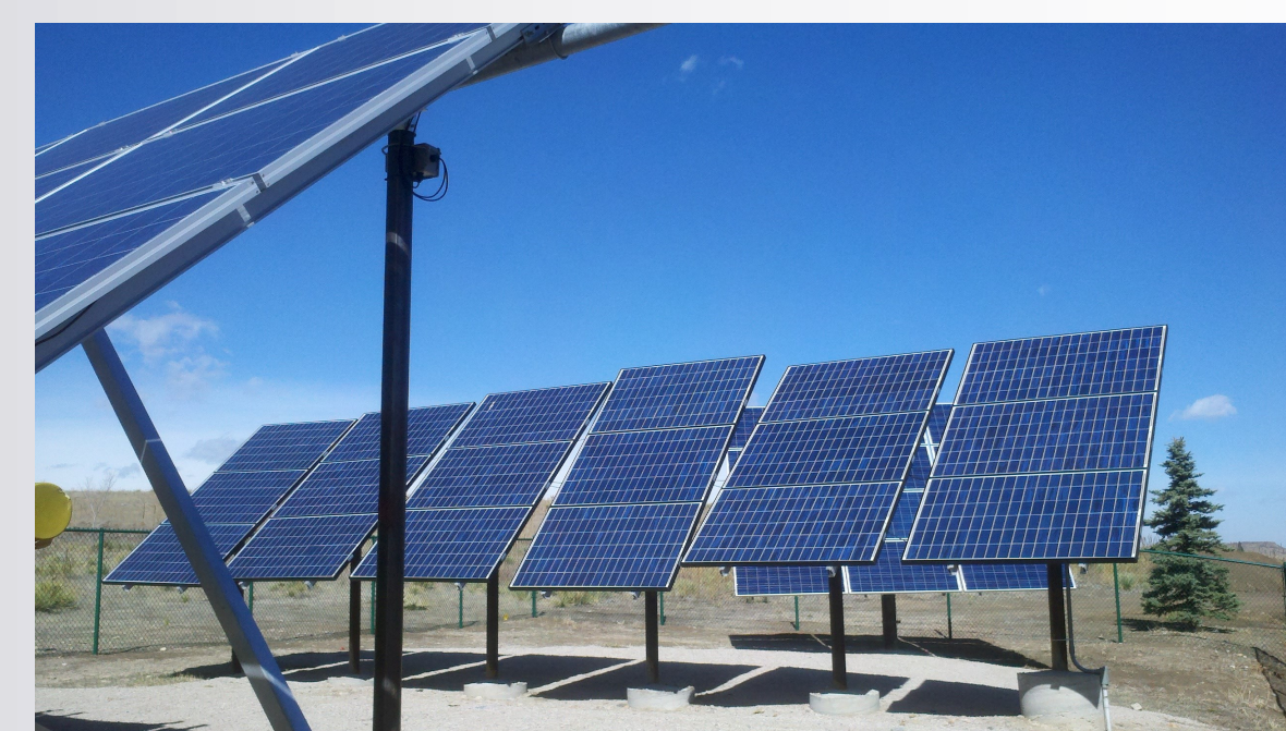
RRCC Solar array that powers our water quality management program building, maintained by our solar energy program students and faculty
