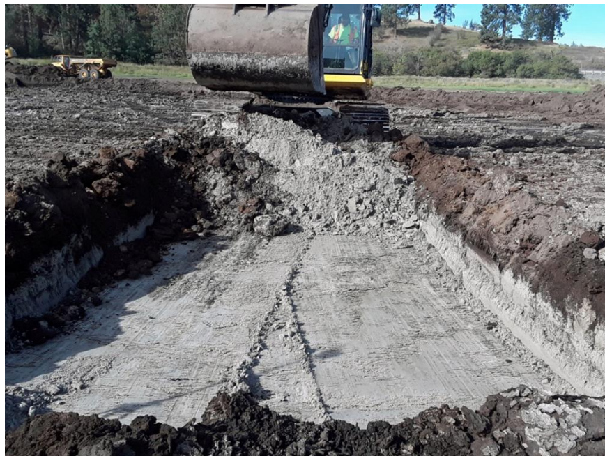
Figure 3. Saltese Flats light-gray ash horizon with initial exposure during excavation of wetland pond.
