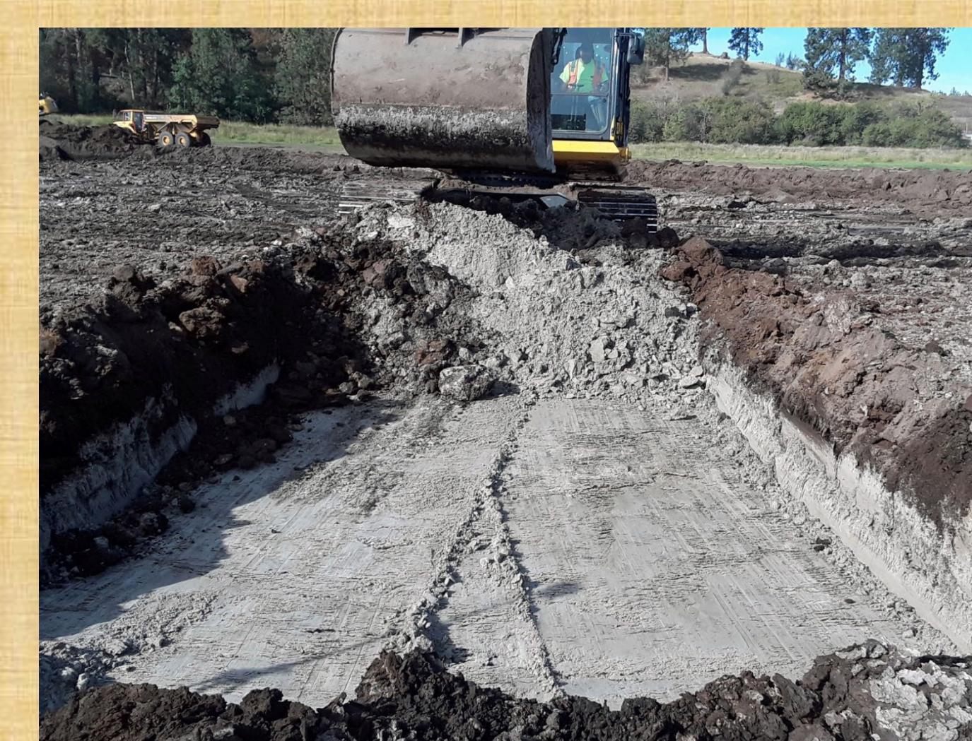
Right: Saltese Flats Mazama ash with initial exposure during excavation of wetland pond. The light gray ash exposed at approximately 1.9 m depth.
