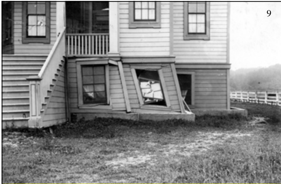
School-house at Point Reyes Station, near Inverness, shifted horizontally two and one-half feet by the earthquake. Photo by G.K. Gilbert.
