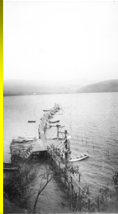
(Right) Post-earthquake photo of Bailey's Pier, Inverness, by GK Gilbert. Originally straight; shifted and much broken. In subsequent repairs, curvature caused by the earthquake was retained.
